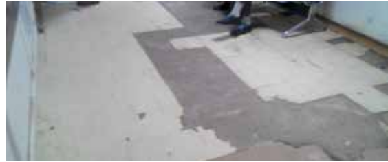
The substandard floor of the accident and emergency section
